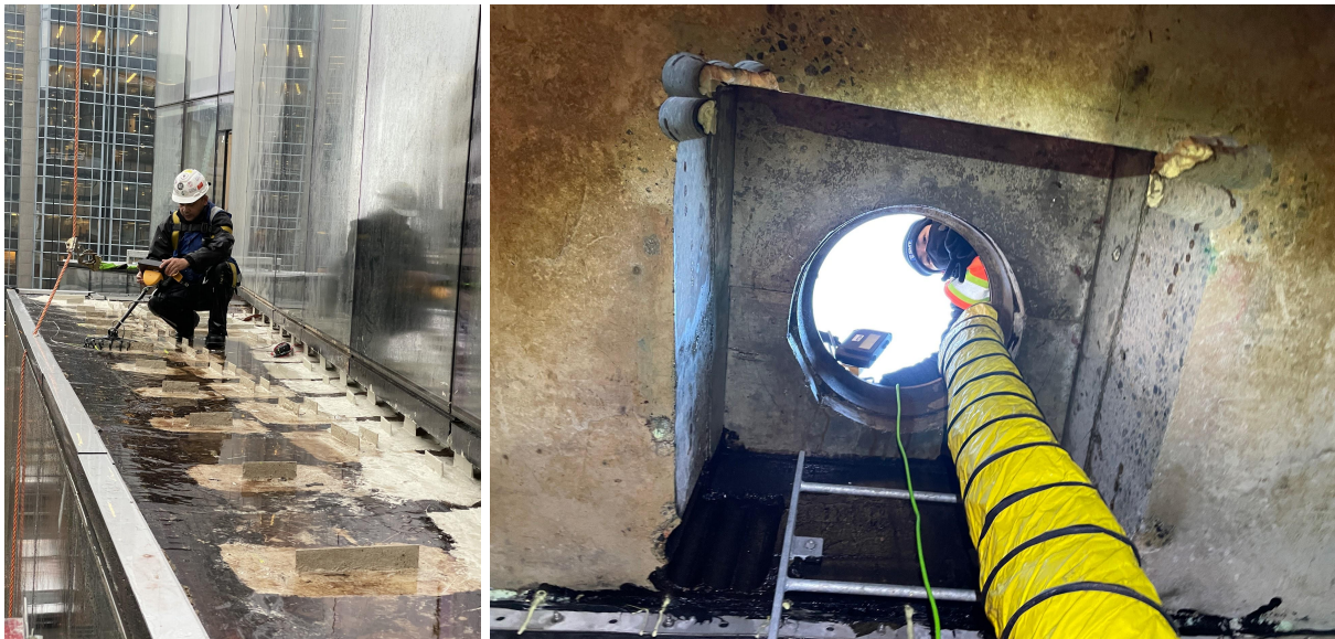
Above Left: SMT Technician uses a harness to scan a high-up ledge.
